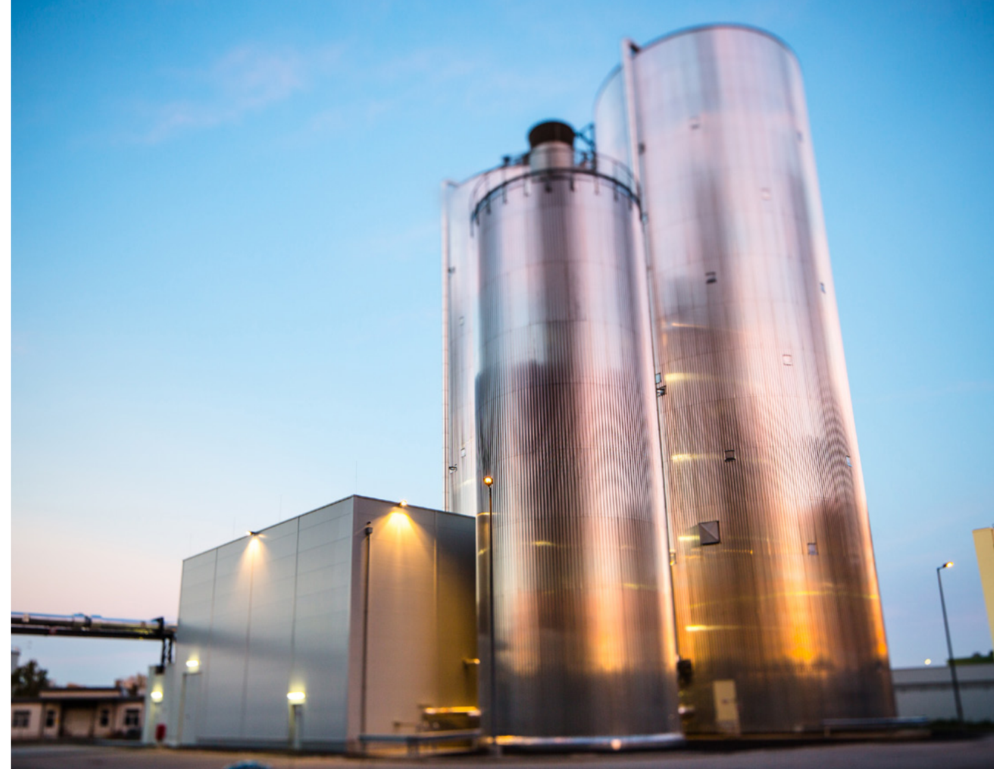
Simmering heat storage tank © Wien Energie_Ian Ehm
